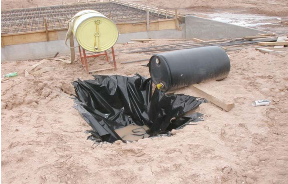
Petroleum Product Storage - Bad
