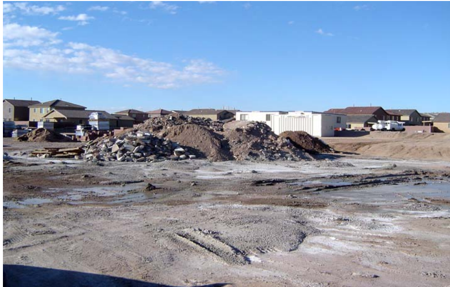
Concrete washout with no containment or sign
