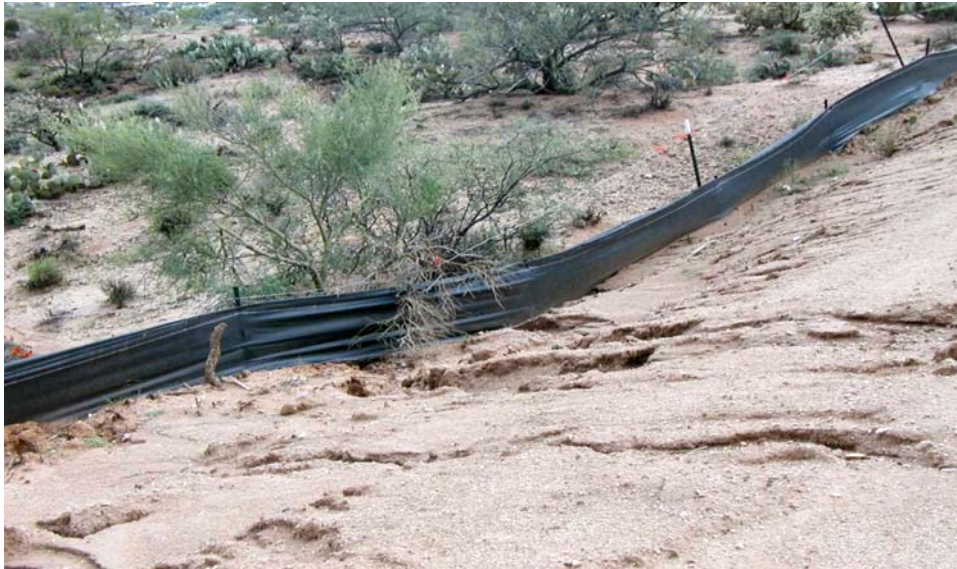
Silt Fence - Bad
