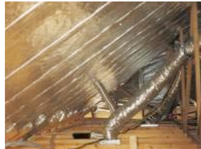
Radiant Barrier - Attic
